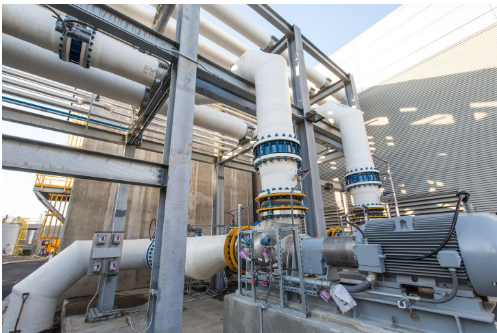
Above: A desalination plant in California. DOE's Advanced Manufacturing Office recently funded 8 projects to undertake innovative research on desalination.
